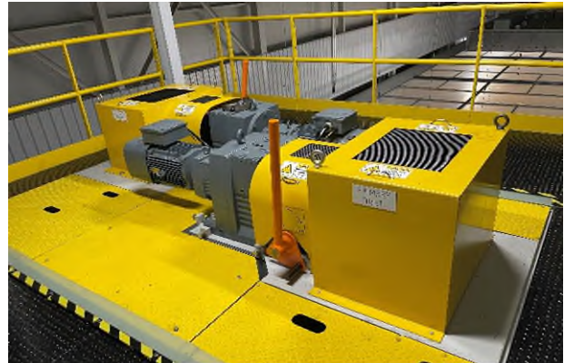
▲ Upper Caterpillar Drive Assembly – Main and Standby Drive Units
