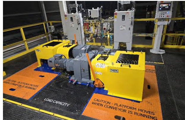
▲ Main and Standby Drive Assembly for ELPO System at GM Lansing Grand River Paint Shop
